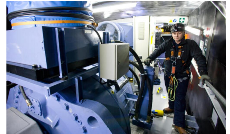
Fig 2 Work area in a Wind Turbine
