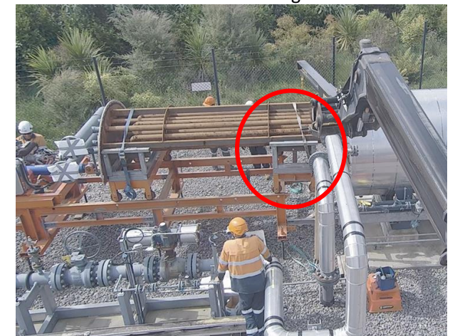
Trolley prior to falling showing position of wheels and tiedown
