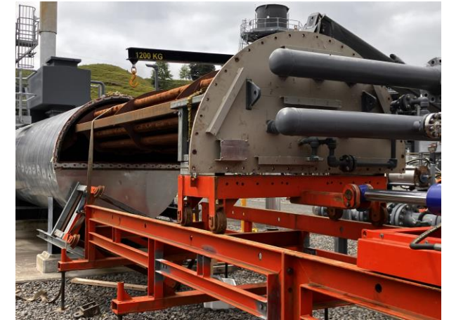
Water Bath Heater Tubing bundle with removal rig
