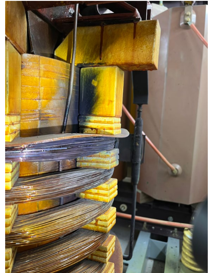
Capillary Tube contacting Tx Windings
