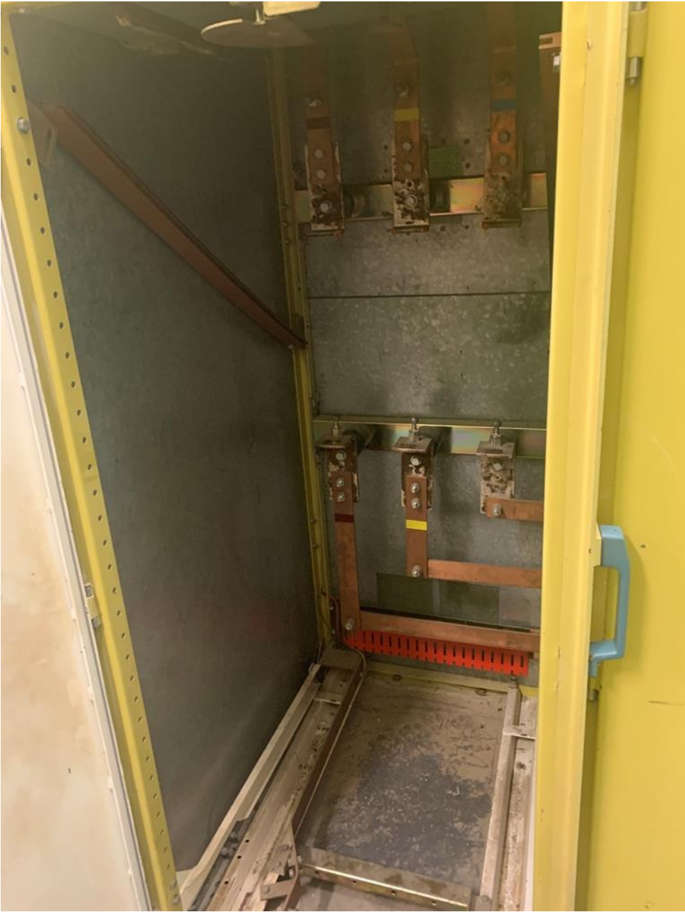
Unprotected 11kV bus
