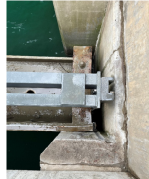
Top view of lifting beam and stoplog in guides
