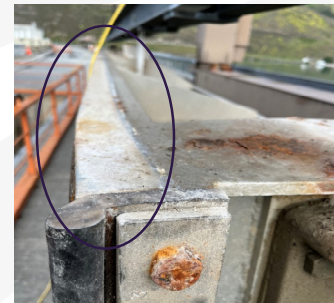
Bent Section of the Stoplog post-event
