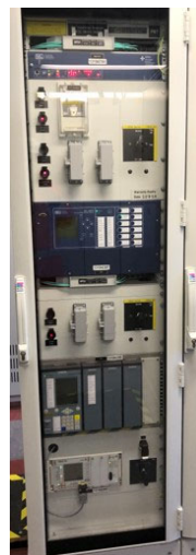
Front Protection Relay
