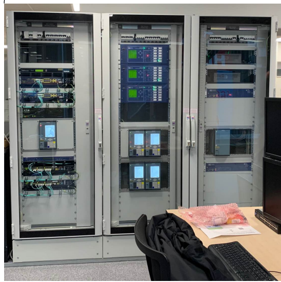
Digital Substation Example
