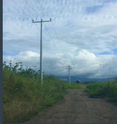
Existing Single Circuit Line
