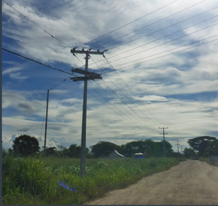
Existing Double Circuit Line
