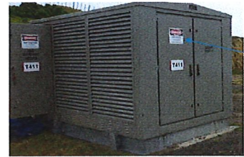
Double access doors with locks
