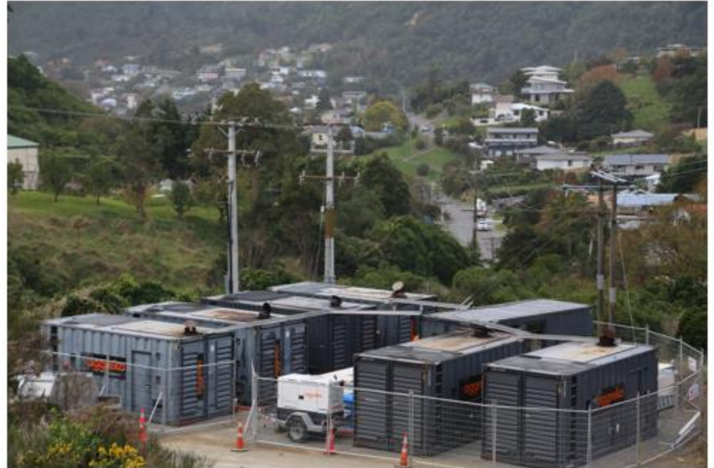
Photo: Generators installed at Scotland Street Quarry
