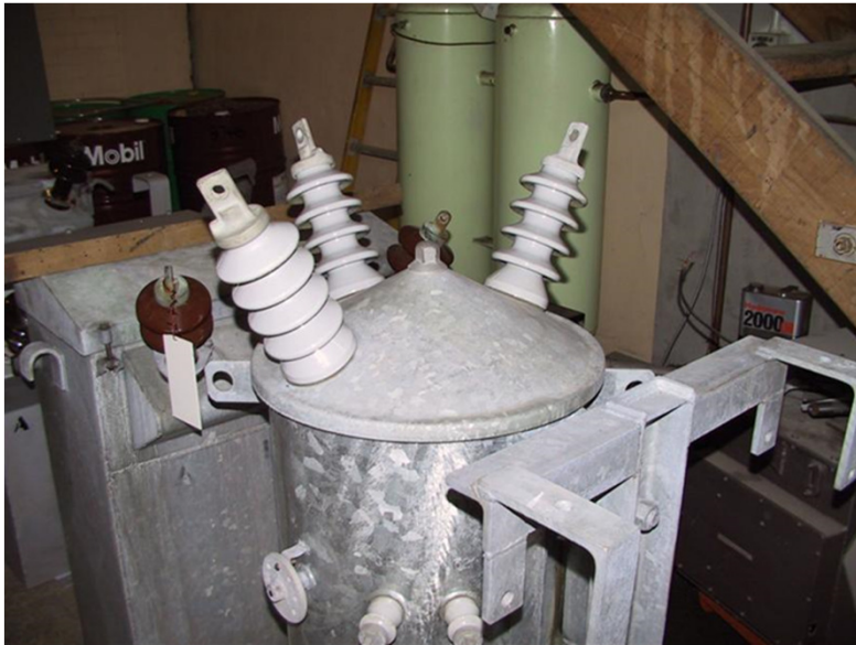
Bushing with problem
